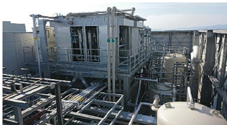
Kumamoto TEC's facility for recovery of water used for gas combustion treatment
