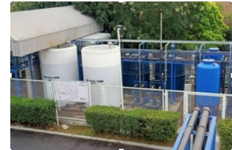
Wastewater treatment recycle plant installed at STT-C
