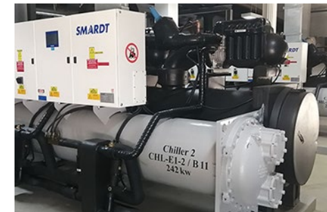
Chiller system installed at STT-C
