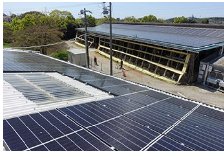
Solar panels installed on cattle barn roofs
