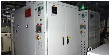
Two-unit plasma abatement system (front unit is on standby; back unit is operating)
