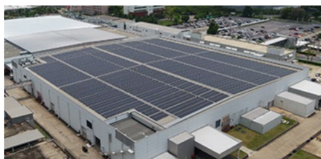
Solar panels on the roof of SDT
