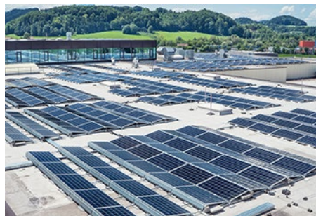
Solar panels on the roof of the Thalgau Plant
