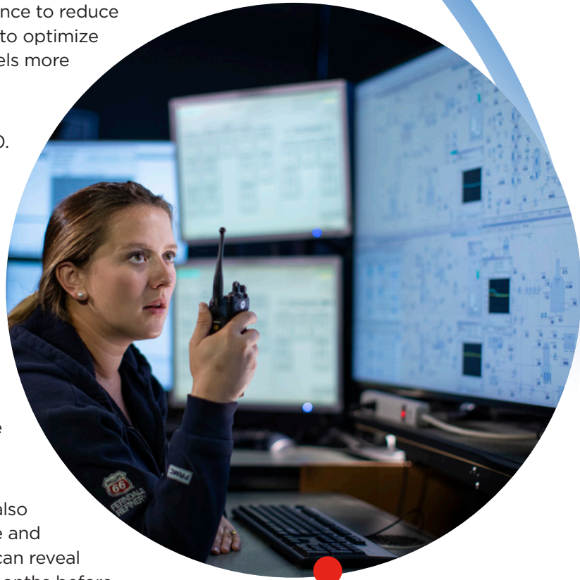
Control room FERNDALE, WA
