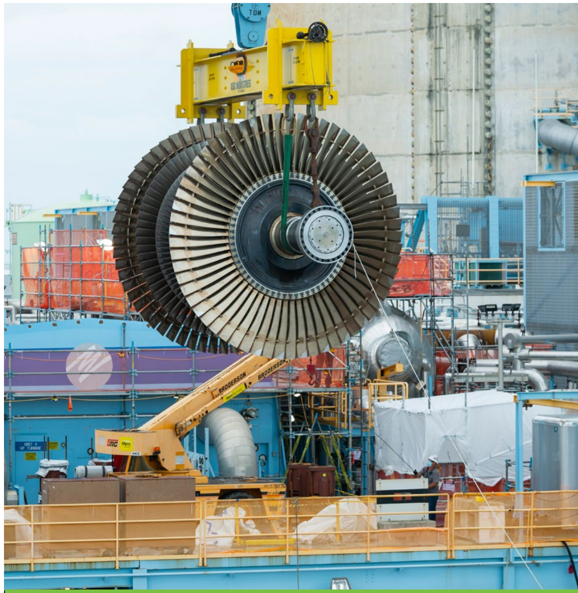
Crews lift a large rotor during a maintenance outage of Unit 4 at the Turkey Point Nuclear Power Plant near Homestead, Florida.
