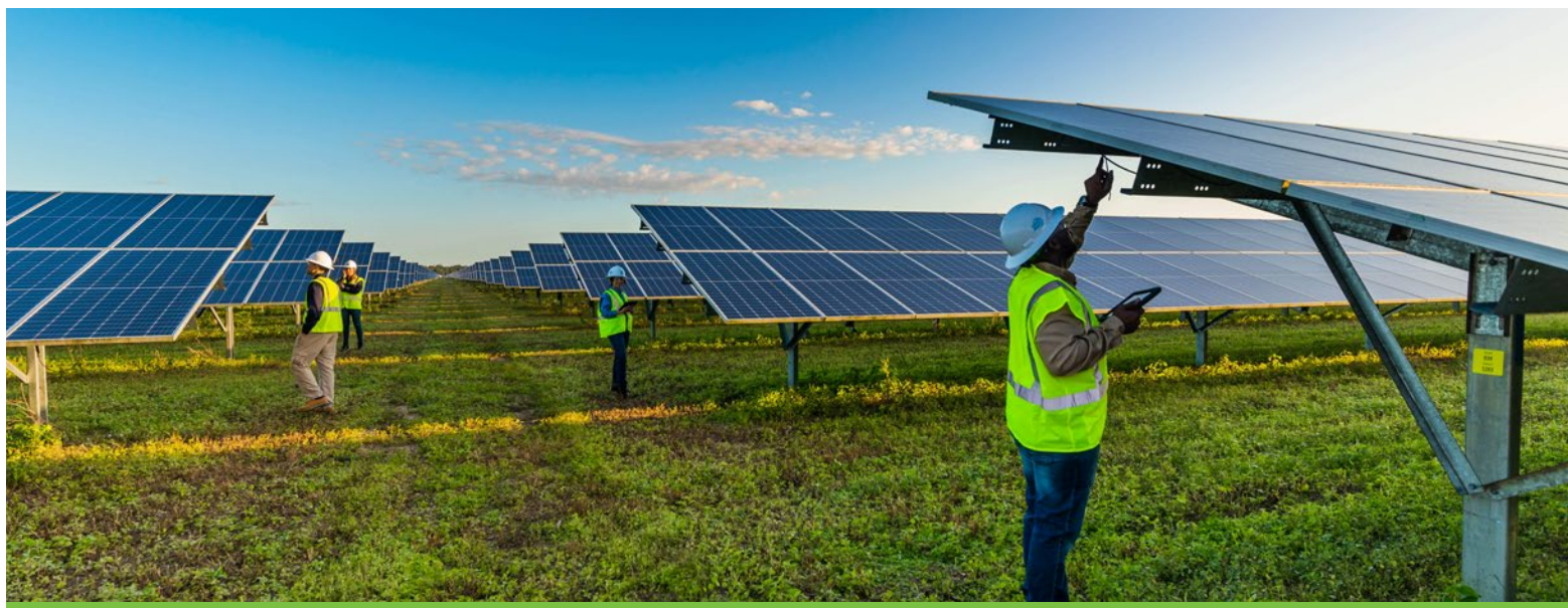
Crews work to commission the FPL Miami-Dade Solar Energy Center in Miami-Dade County Florida.
