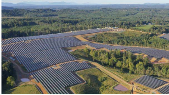
61.6 MW Altavista Solar Project in Virginia
