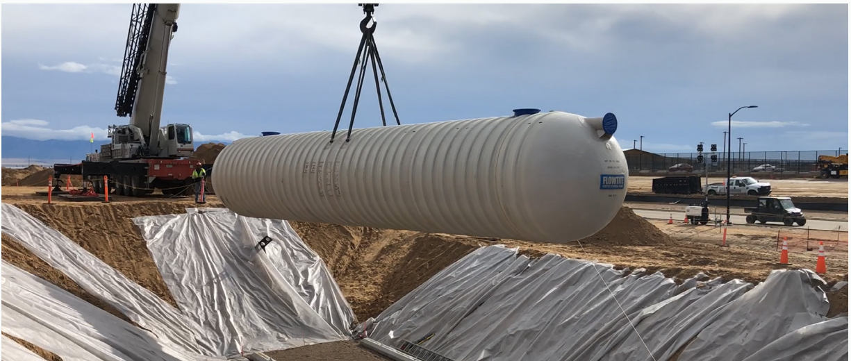
For our Los Lunas, New Mexico data center located in a desert climate, we engineered a system that captures rainwater from the roof in an underground cistern and cuts in half the amount of potable water needed to irrigate the surrounding campus landscape.
