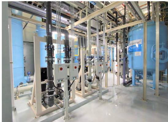
Fab 18A biological treatment system.
