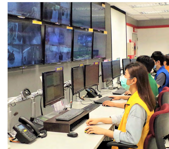
Facility Monitoring & Control Center.
